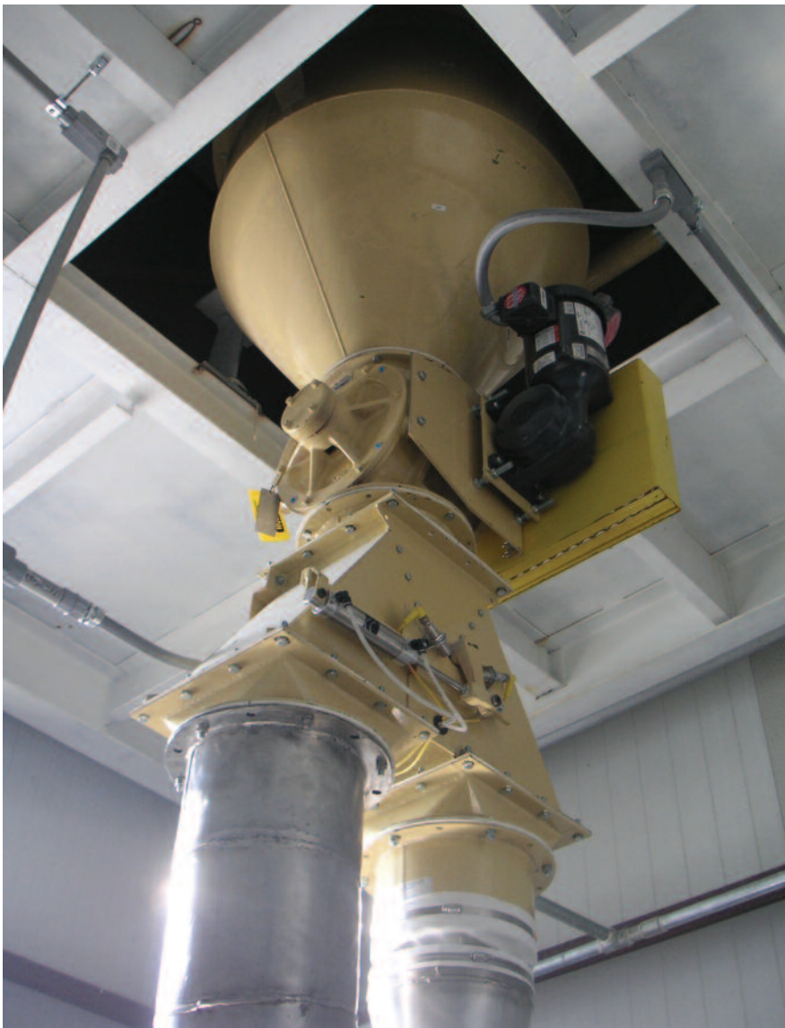
The automated control system remotely actuates a storage silo’s diverter valve to direct the corn kernels to the appropriate processing line.
