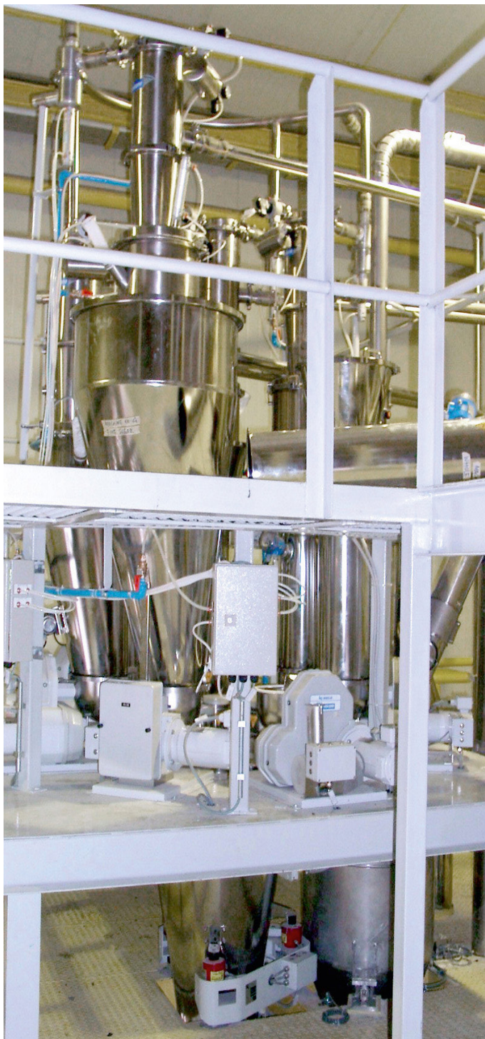
Gain-in-Weight batching station for a bakery installation
