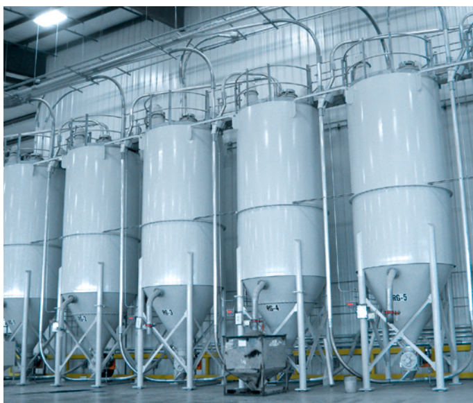
Coperion K-Tron pneumatic conveying system
