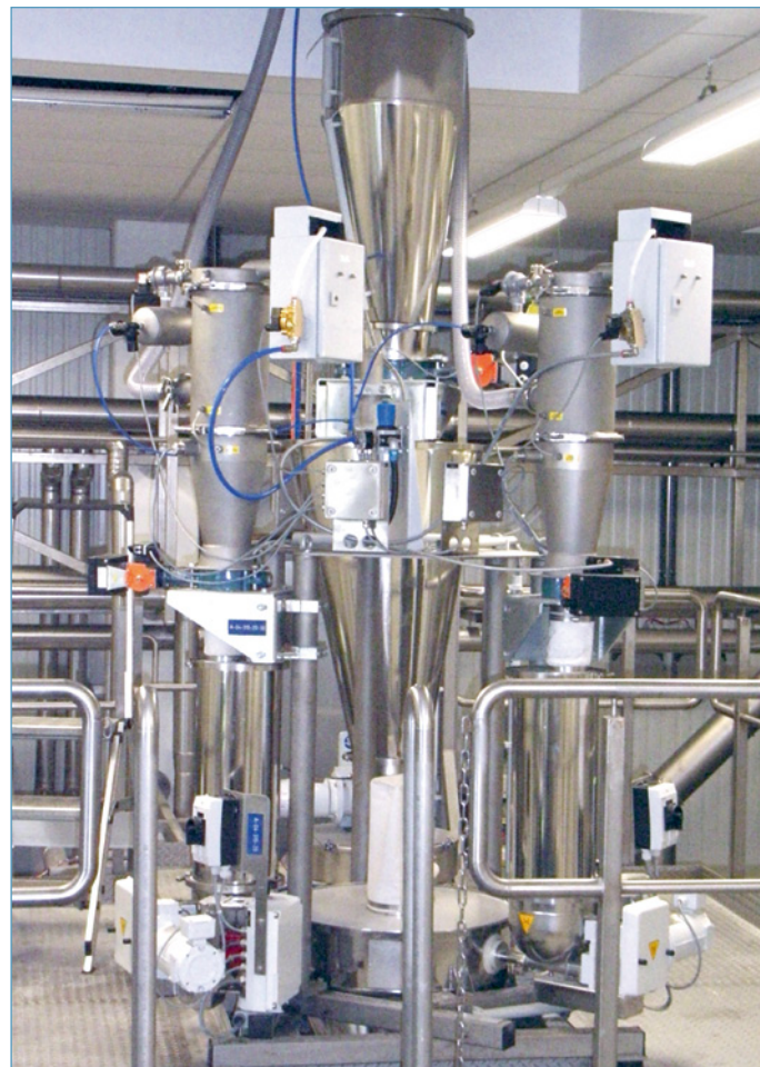
Fig. 4: Gain-in-weight batching system in a food application
